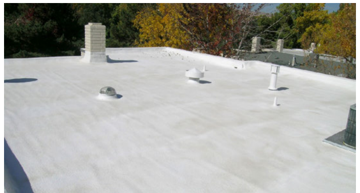
Cool roofing material
