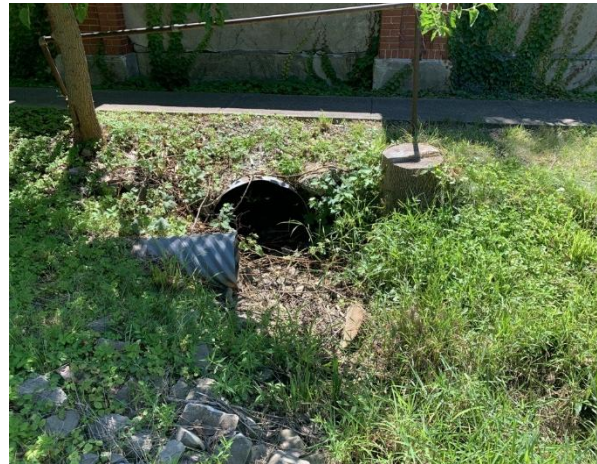
Photo 12 – Downstream extent of Reach 3, where it flows under a wall, under John Street East, and into a roadside ditch.
