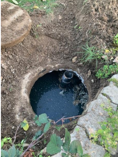
Septic Tank – Secondary Chamber
