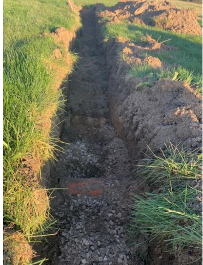
Existing Clay Distribution Pipes
