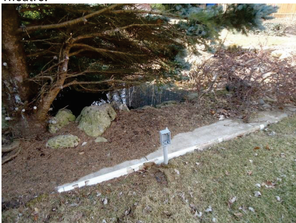
Plate 5: Edge of filled in former pool beside pond; note buried electrical.
